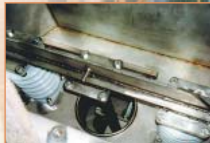
Hardware Improvements for Enhanced Reliability
